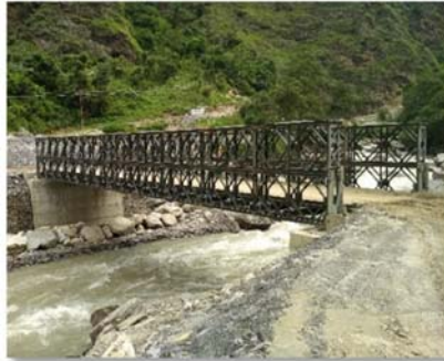
100 feet span Bailey bridge erected on a rural road project at Solukhumbu District
