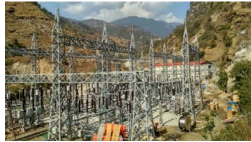
Likhu A Switch Yard
