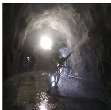
Shot concrete in progress for Tunnel support Tunnel Face drilling in progress
