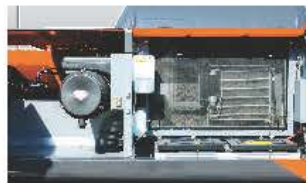
Utility space and radiators
